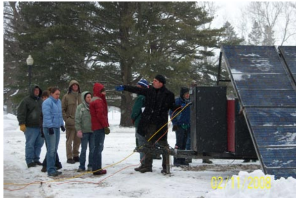
Prof. Gamble hooks up the solar panels to Goodnow Hall with the students help.
